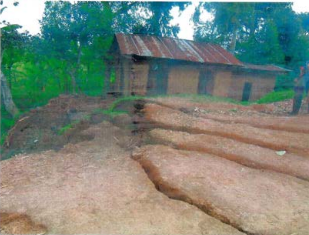
House at risk
