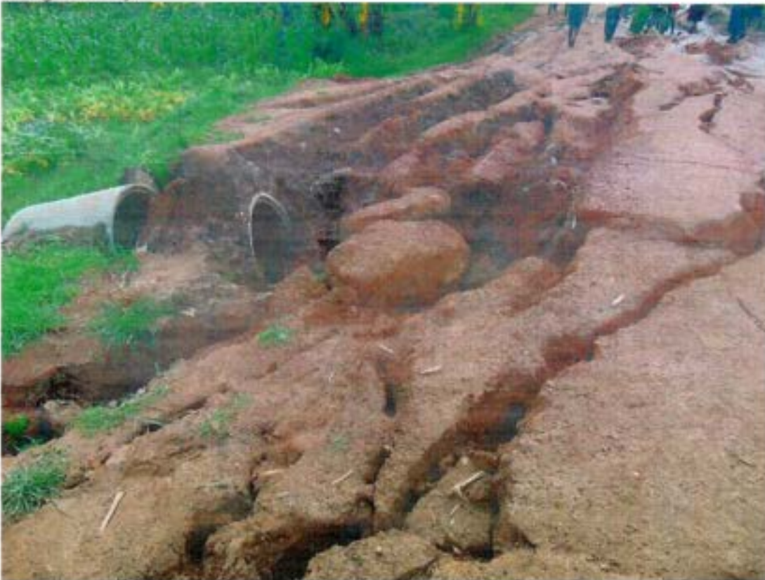
Buputo to Magale road destroyed
