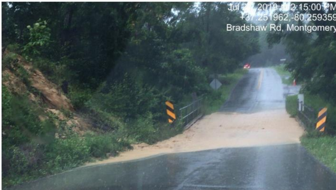
Figure 5. Sediment laden runoff flowing across Bradshaw Road into Bradshaw Creek.
