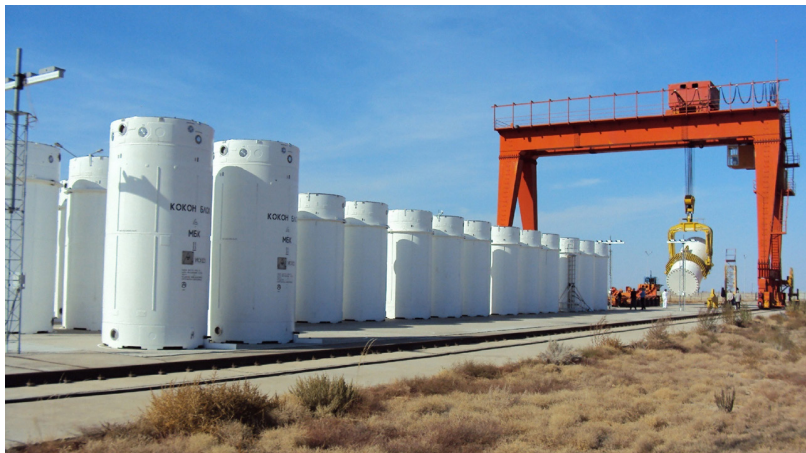
At right, a dry storage cask recently loaded with spent fuel is lifted from a horizontal transporter to be placed on a specially designed storage pad. (Courtesy: Sandia National Laboratories)
