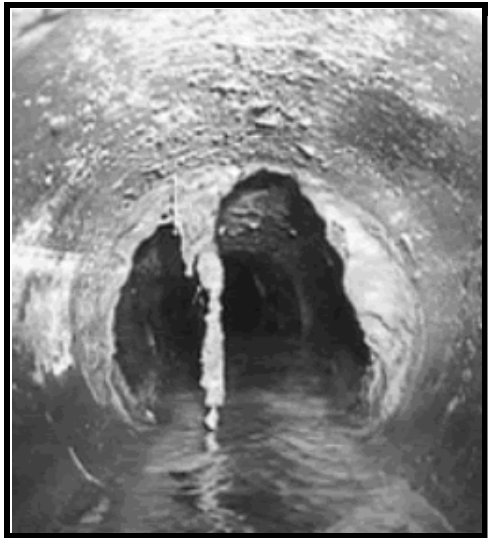
Root and grease buildup can cause blockages in a sewer system [photo: North Carolina Department of Natural Research (NCDNR)].
