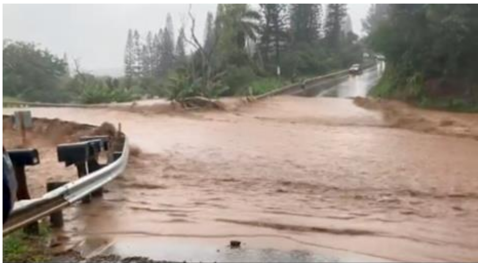
Flooding on Hana Highway. Id.
