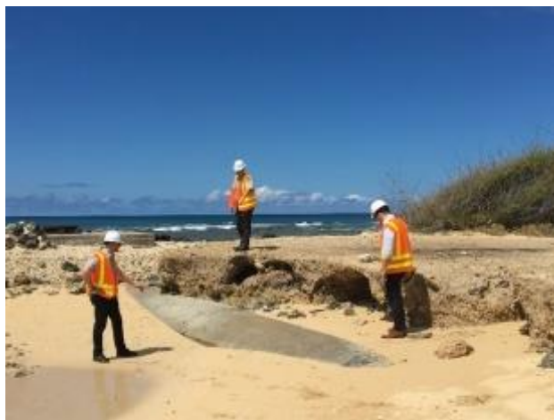
Sea level rise creates conditions for rapid erosion at the Sand Island Wastewater Treatment Plant, meaning overnight exposure of the outfall pipe. City and County of Honolulu, Office of Climate Change, Sustainability and Resilience.
